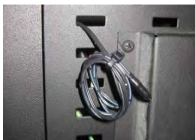
Figure 22 - Room temperature probe
