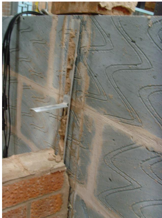
Plate 2 Deformation of Channel -Wall 2
